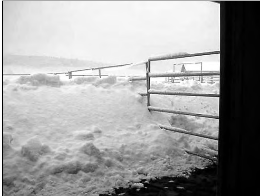
Several horses were trapped inside, and a few outside, this barn after four feet of snow slipped off the metal roof. Thankfully none was injured. Caution is advised for all owners, especially those with older or slipshod shelters.
