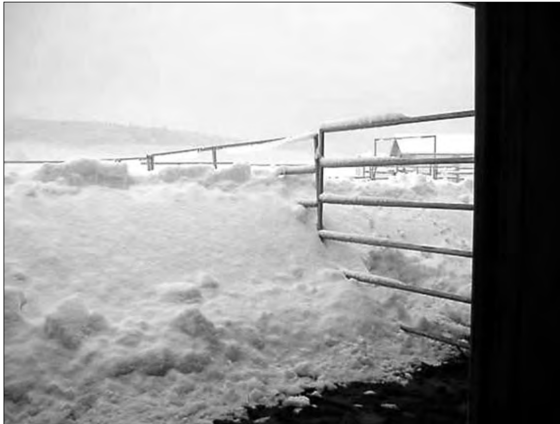
Several horses were trapped inside, and a few outside, this barn after four feet of snow slipped off the metal roof. Thankfully none was injured. Caution is advised for all owners, especially those with older or slipshod shelters.
